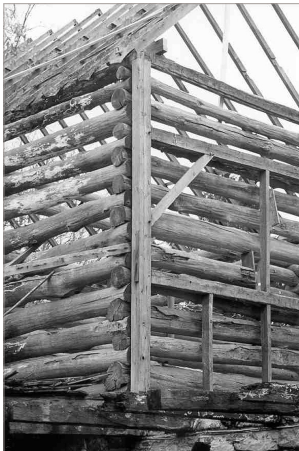
Photo of the historic Jones Log Barn as it was dismantled for rebuilding as the 'Living History Center at Duportail'.
